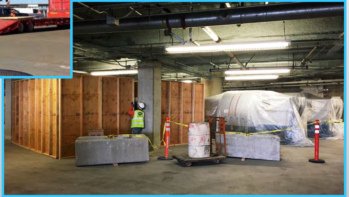
TSA delivery of eight baggage screening machines
